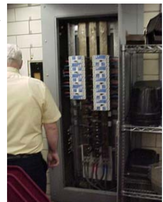
Figure 2a: Electrical panel with missing dead front
