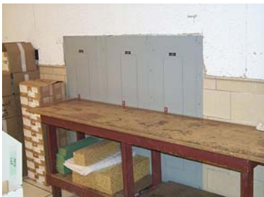
Figure 1: Blocked Electrical Panel
