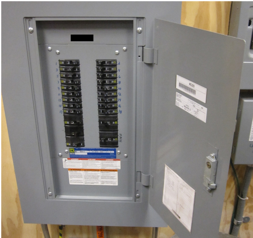
Example of an enclosed electrical panel.
