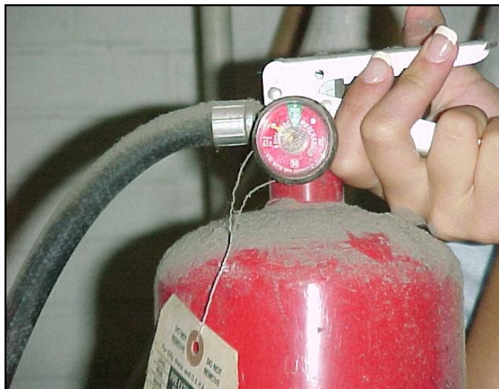
Figure 3: Extinguisher with insufficient pressure
