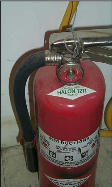
Figure 2: Halon fire extinguisher
