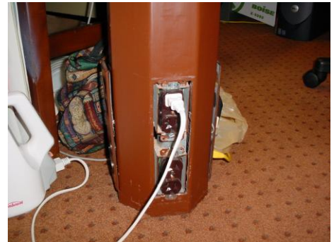
Picture 2 Faceplate missing from outlets
