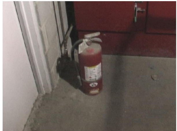
Picture 6 Unsecure fire extinguisher
