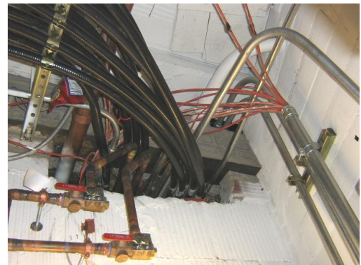
Picture 5 Penetration in a fire wall
