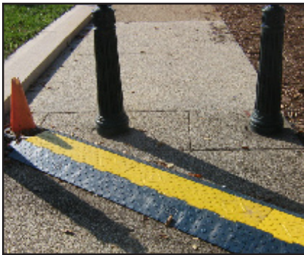
Figure 1: Non-compliant temporary sidewalk ramp
