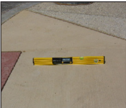
Figure 2: Non-compliant newly installed sidewalk curb cut
