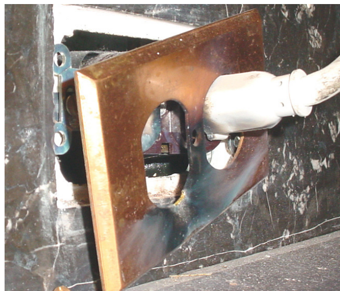
Broken and burnt outlet
