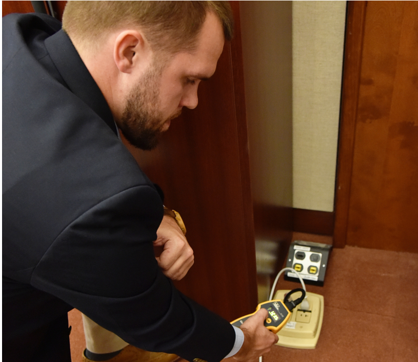
OOC OSH Specialist using a circuit analyzer to measure impedance.
