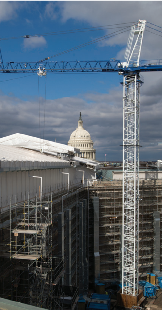
Phase I of the Cannon Renewal Project began in January 2017. Credit: Architect of the Capitol.
