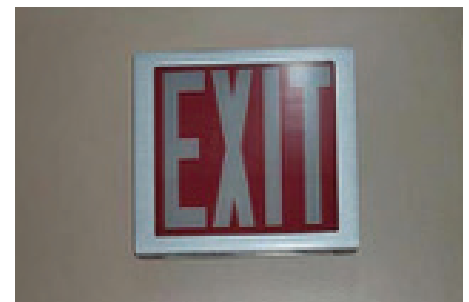
Figure 2: An externally illuminated Exit sign
