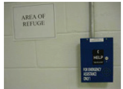
Figure 6: Push-to-talk two-way communication box with temporary “Area of Refuge” sign
