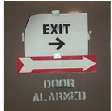
Figure 1: Improper paper Exit sign
