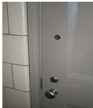
Figure 3: Hole Through Fire Door
