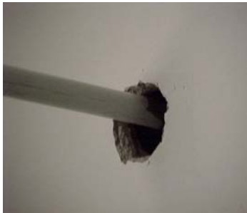
Figure 1: Pipe Poking Through a Fire Wall
