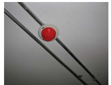
Figure 2: New Smoke Detector
