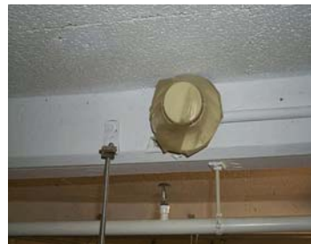
Figure 1: Covered Smoke Detector
