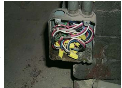
Figure 2: Potentially hazardous wall switch or outlet box without cover
