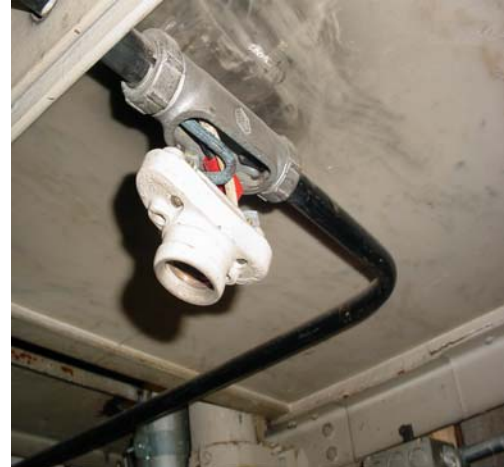
Figure 6: Light fixture not properly secured to mounting with open socket and exposed wiring
