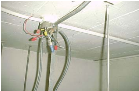
Figure 1: Potentially hazardous electrical junction box without cover
