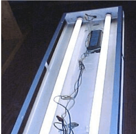
Figure 5: Missing cover on fluorescent light fixture exposes wiring
