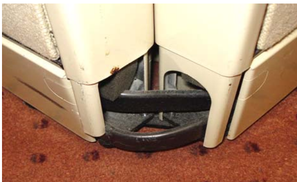
Figure 7: Exposed power wiring at corner unprotected from impact and damage
