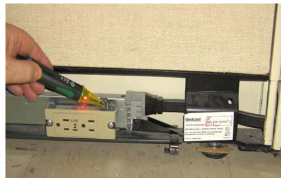
Figure 8: Exposed baseboard electrical supply outlet and service without its cover
