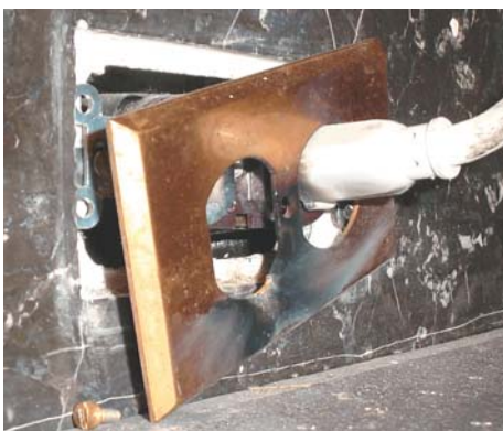
Figure 3: Potentially hazardous burnt outlet with displaced cover
