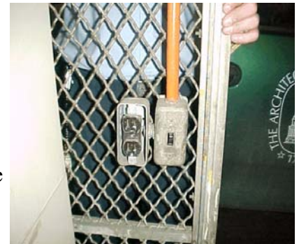
Figure 4: Potentially hazardous outlet with no cover next to switch
