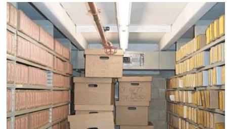
Figure 1: Stacked materials too high blocking sprinkler's range.
