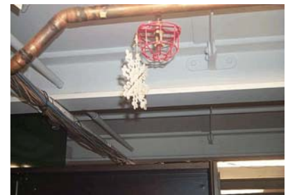
Figure 3. Decoration hanging on sprinkler guard.
