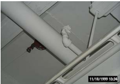
Figure 2 Completely covered sprinkler
