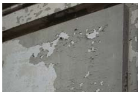
Figure 3: Removal or encapsulation is necessary when extreme lead paint flaking occurs.
