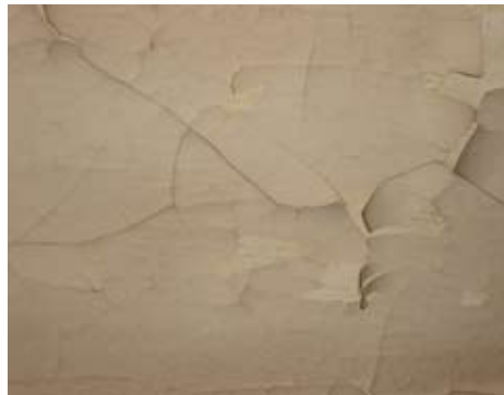
Figure 2: While top paint coats may not contain lead, under layers may have high lead content.
