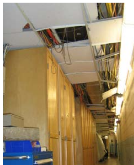
Figure 2: Removal of ceiling tiles may damage wiring to detectors mounted below them.
