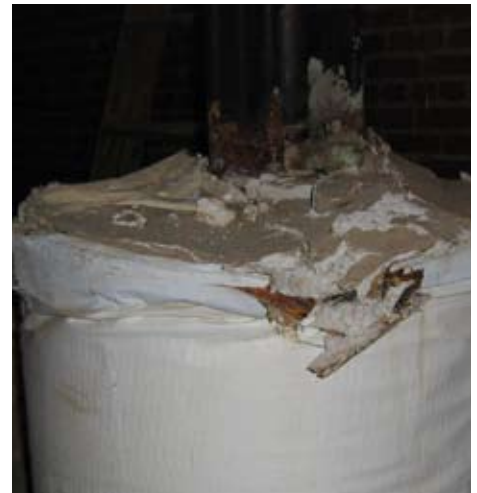
Figure 2: A damaged pipe insulation jacket exposes friable asbestos.
