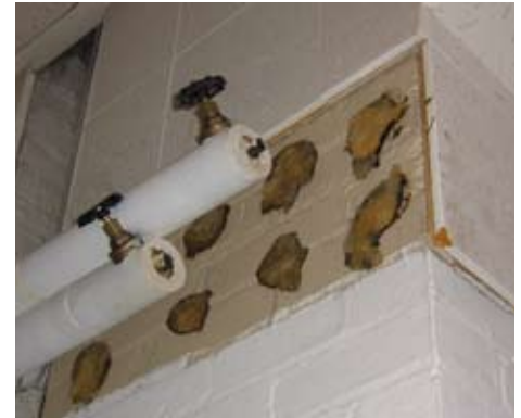
Figure 1: Damaged 9-inch vinyl tile exposing mastic
