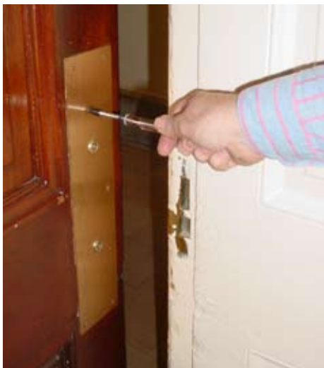
Image 1: The force required to open this door is too great.
