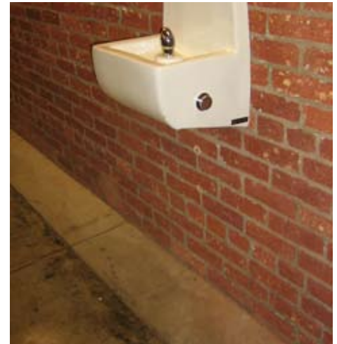
Image 2: Leading edge on this water fountain is too high: more than 27 inches above the floor.
